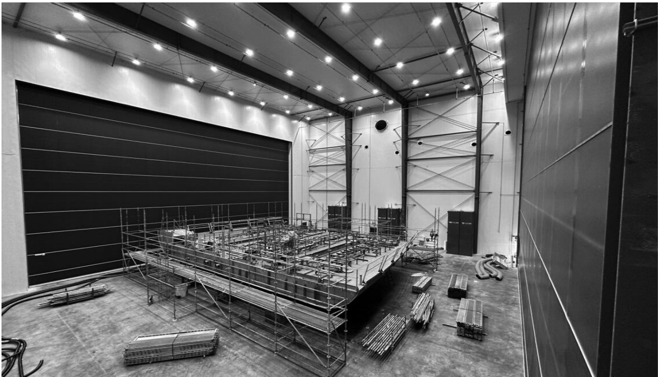
Fig. 5, Blast and Paint Booth with Middle Door View 1
